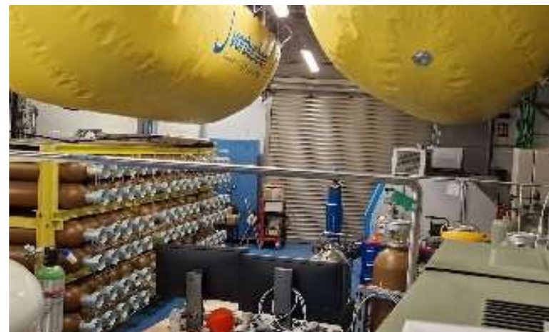
Helium recovery plant
